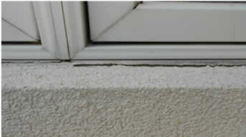
Caulk failing (typical)
