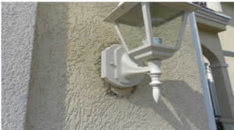
Light fixtures need to be caulked (typical)
