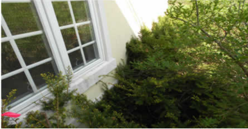
Bushes should be cut back away from the EIFS system (typical)
